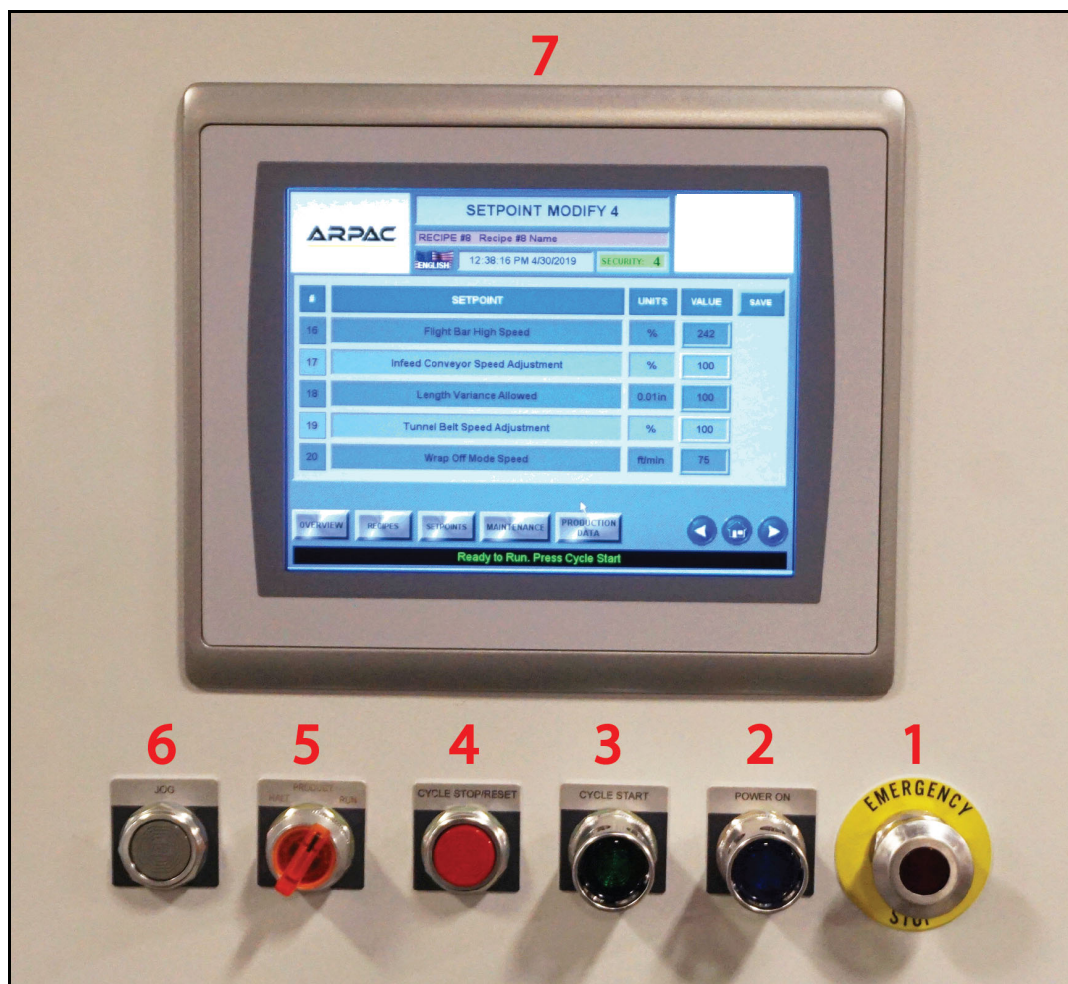
Figure 4-2 - Wrapper Main Control Panel
