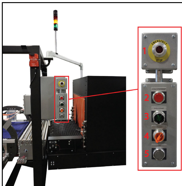
Figure 4-4 - Auxiliary Control Panel 3
